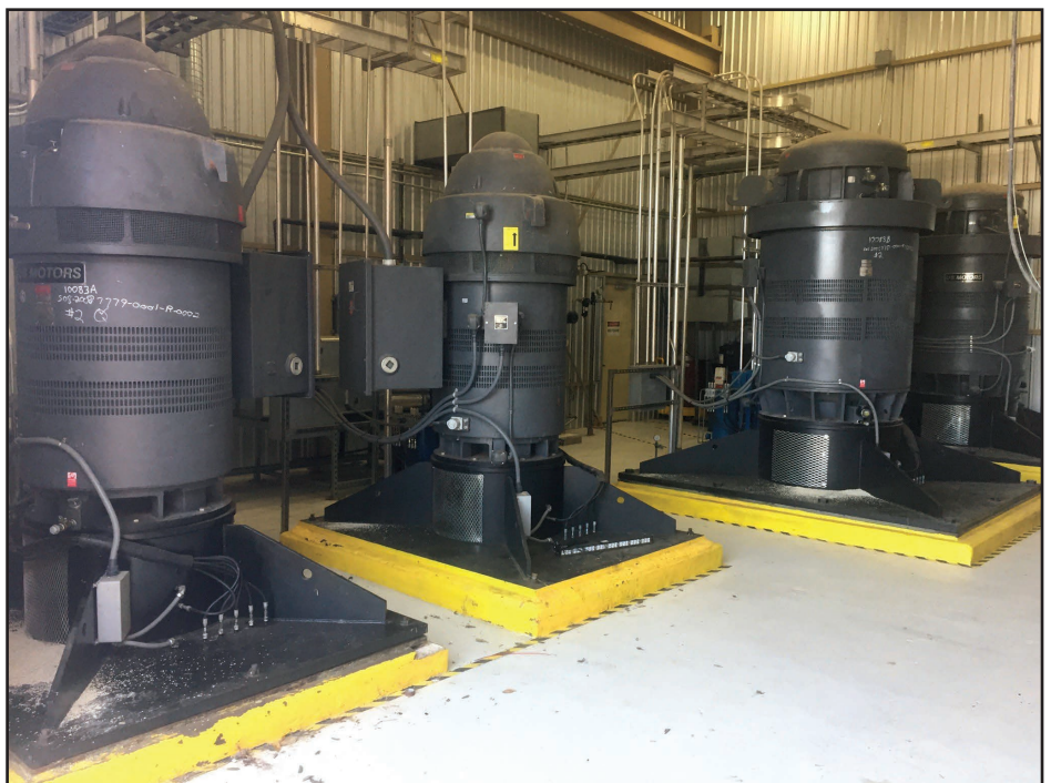
FBC LID 2 Storm Water Pumps
