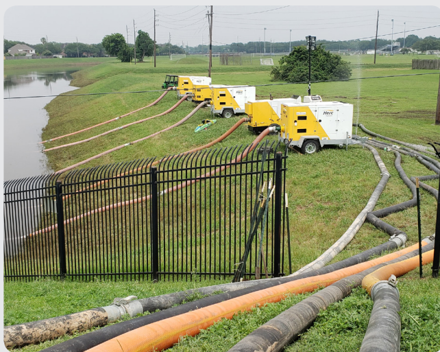
Auxiliary pumps brought in to help pump water out of the levee
